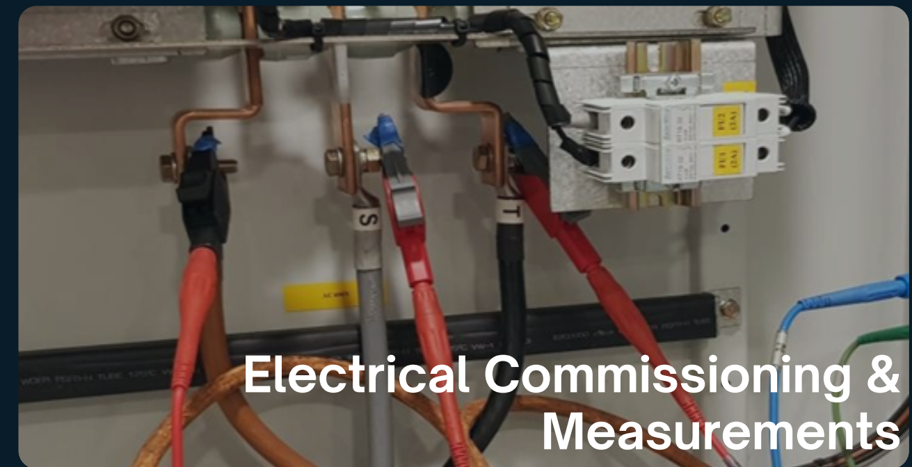
Power Supplies & VFD Installations
